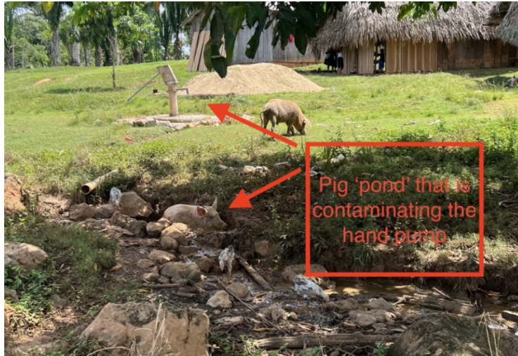
Figure 32: Foraging Pigs contaminating the Hand Pumps in Otoxha (Source: Site visit, 2023)
