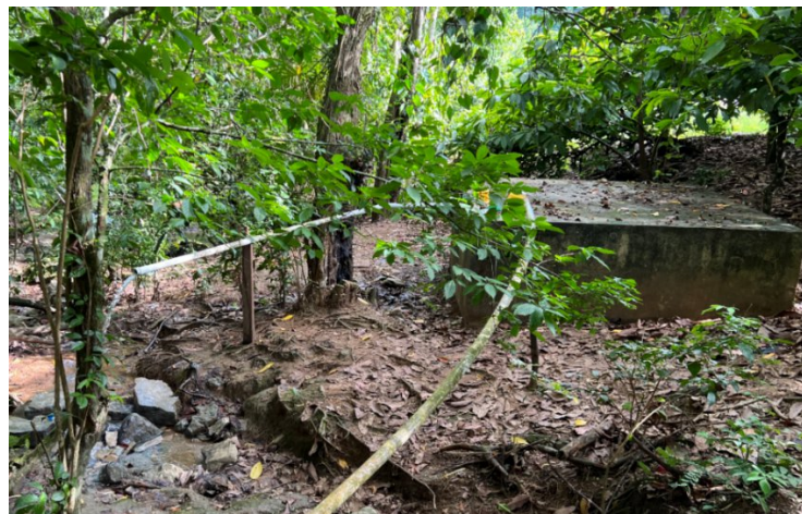
Figure 34: Spring Water Reservoirs with PVC Pipes to the Village (Source: Site visit 2023).
