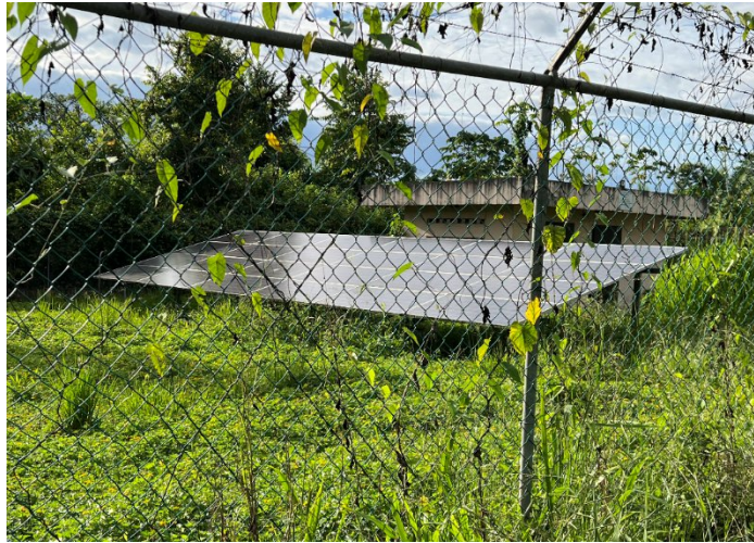
Figure 22: Example of Solar Panels used for Water Pump (Source: Site visit 2023).
