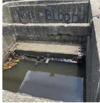
Figure 13 Matanimoli and Navaka village have floodgates that was built in 1990s and need repair to protect the village against flooding
