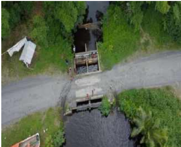
Figure 12 Vuci village and the existing 2-barrel flood gate which needs repair through replacement of steel gates.
