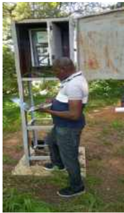
Hydromet Station (CHAD)
