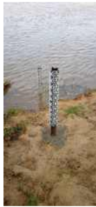
Water level gauge
