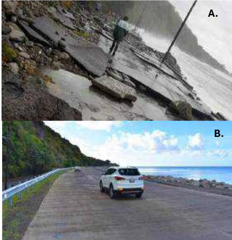
Figure 12: A.) Damaged main road in Old Road Bay after the passage of Hurricane Maria in 2017, B.) Repaired Road in Old Road Bay in 2021, showcasing post-disaster recovery efforts.
