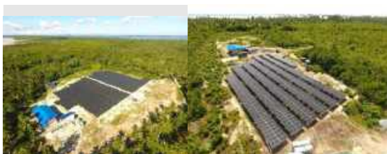
Figure 22. Photovoltaic plants and diesel generators deployed by the RETS project in Sibutu and Sitangkai, as of October 2021. Source: The RETS project
