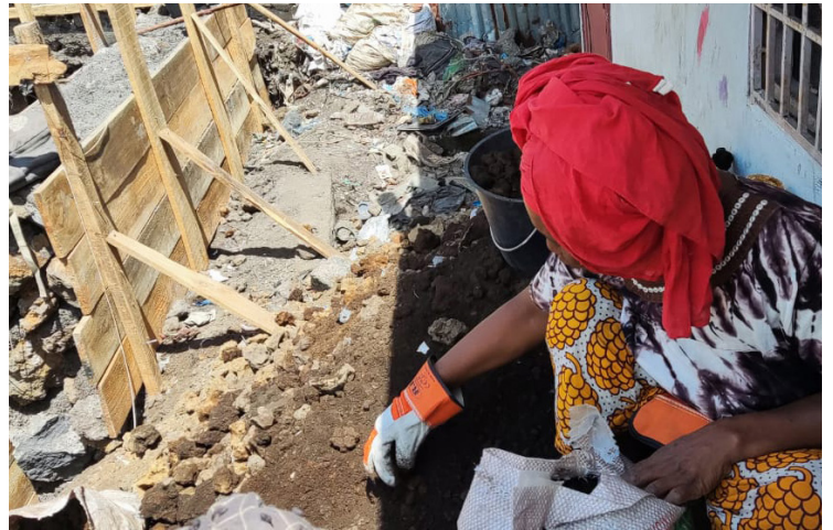
Community members in La Coulée, Moroni, help construct rainwater tanks, improving water access and reducing flood risks. (Photo by Oxfam)
