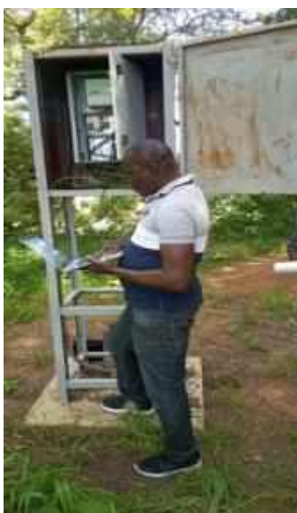
Hydromet Station (CHAD)
