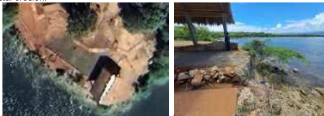
Figure 6. Admiral's House in La Isabela National Park. Google Earth aerial view from December 2023 (left) and photo taken in April 2024 during the proposal origination mission (right). Approximately one-third of the house enclosure has collapsed due to coastal erosion.
