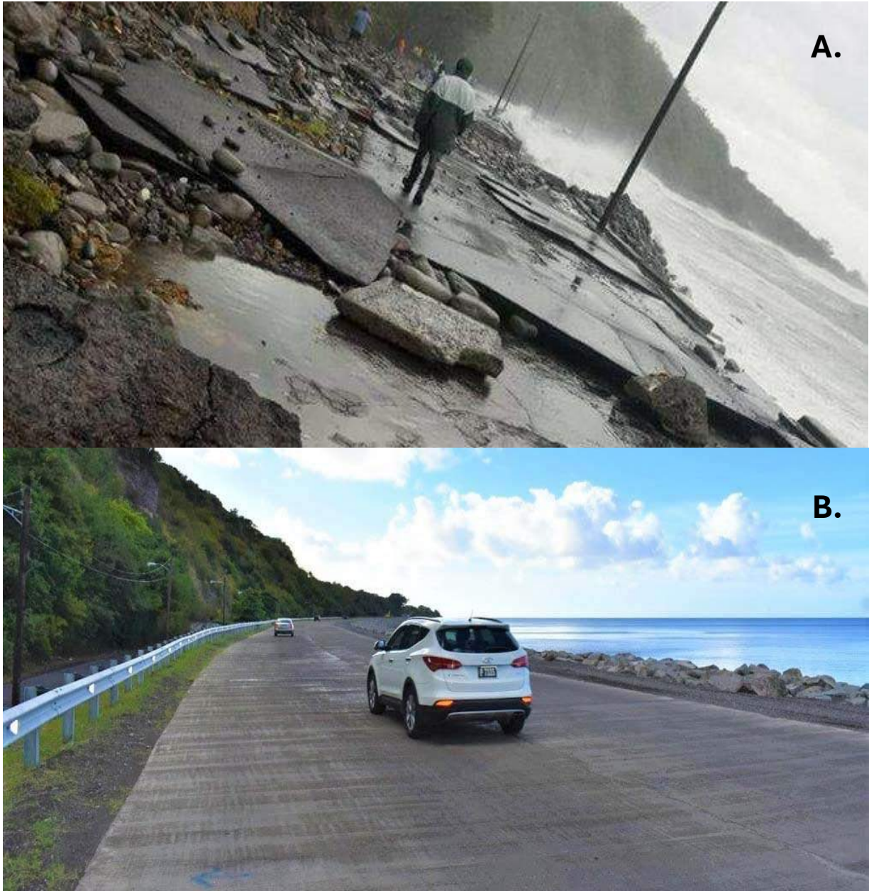
Figure 12: A.) Damaged main road in Old Road Bay after the passage of Hurricane Maria in 2017, B.) Repaired Road in Old Road Bay in 2021, showcasing post-disaster recovery efforts.
