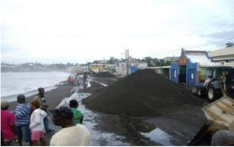
Figure 14: An impassable and severely damaged Irishtown Bay Road in the aftermath of Hurricane Omar (2008)
