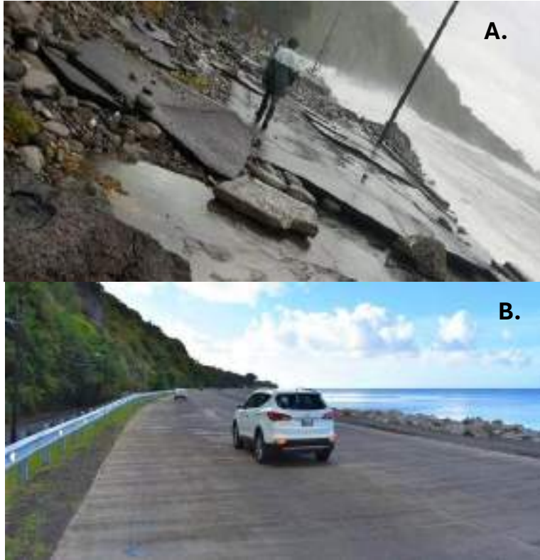
Figure 12: A.) Damaged main road in Old Road Bay after the passage of Hurricane Maria in 2017, B.) Repaired Road in Old Road Bay in 2021, showcasing post-disaster recovery efforts.
