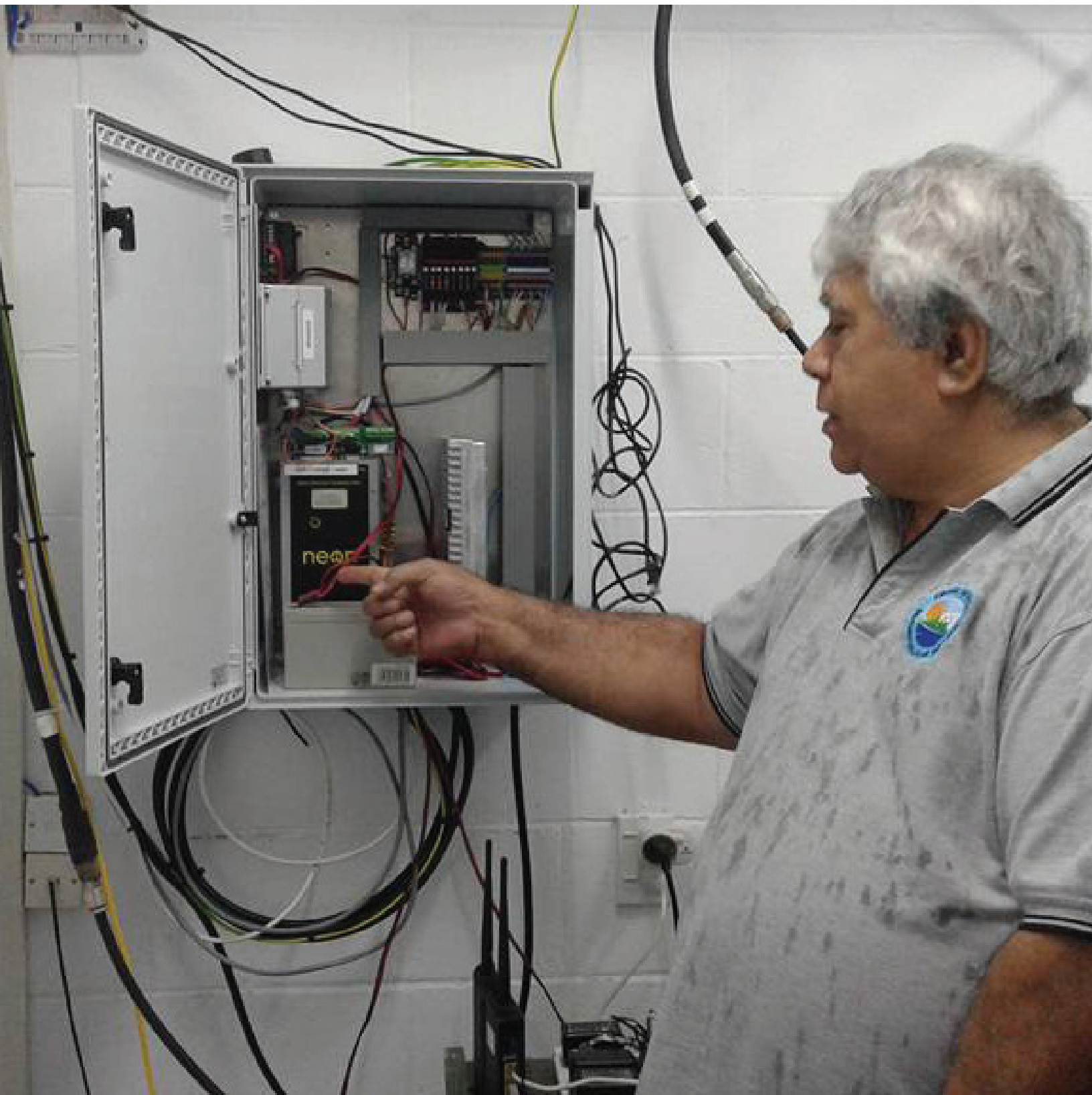
Early Warning Systems (EWS) technician showcasing the server room, Cook Islands Photo by Melina Tuiravakai
