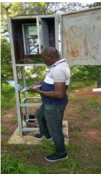
Hydromet Station (CHAD)
