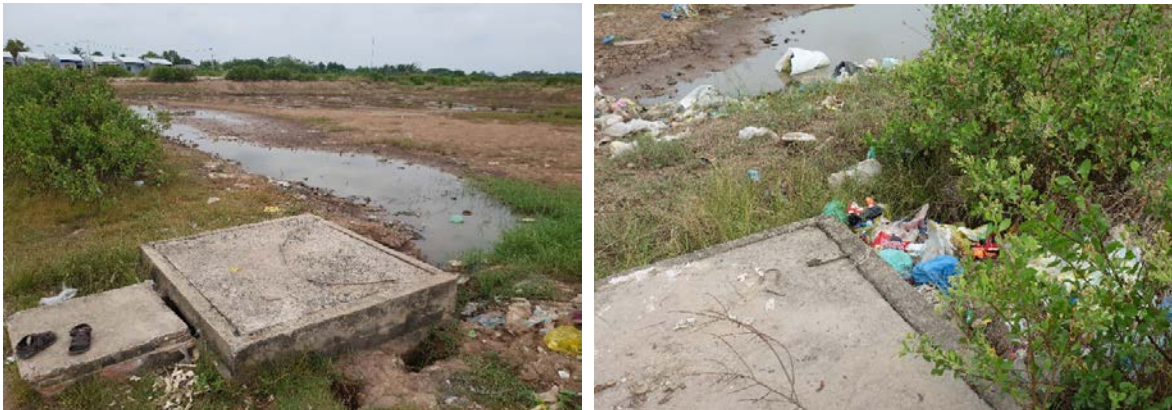
Figure 12. Water drainage system
