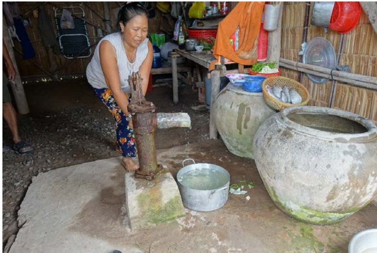
Figure 23. Water pumping system in the household
