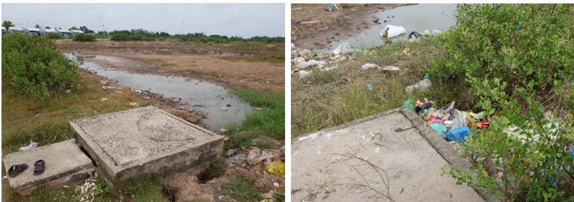
Figure 12. Water drainage system
