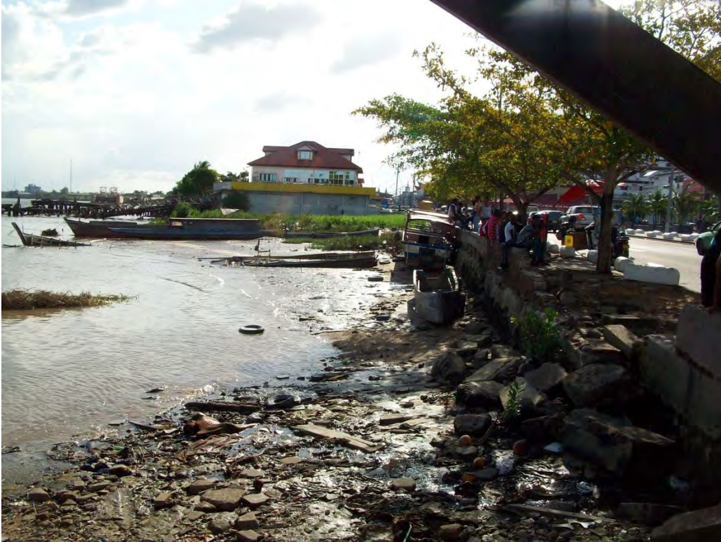
Figure 31: Existing Historic Flood Protection Wall – Note Extensive Disrepair
