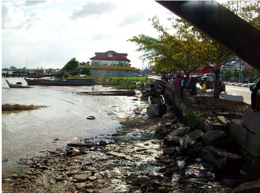
Figure 3-2: Existing Historic Flood Protection Wall - Note Extensive Disrepair
