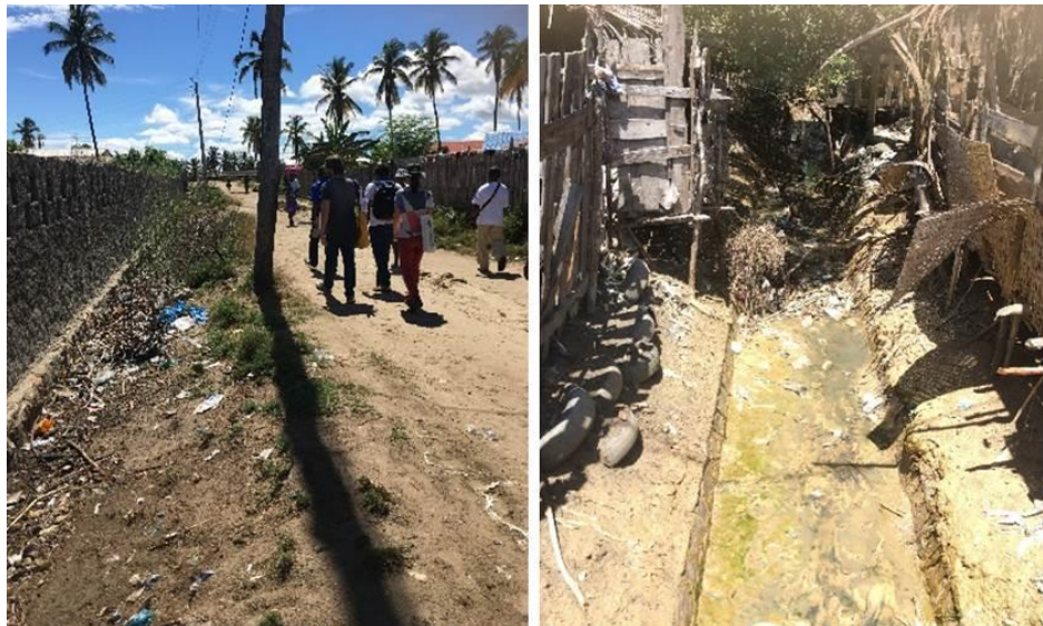
Figures 15 and 16: Drainage conditions in Morondava
