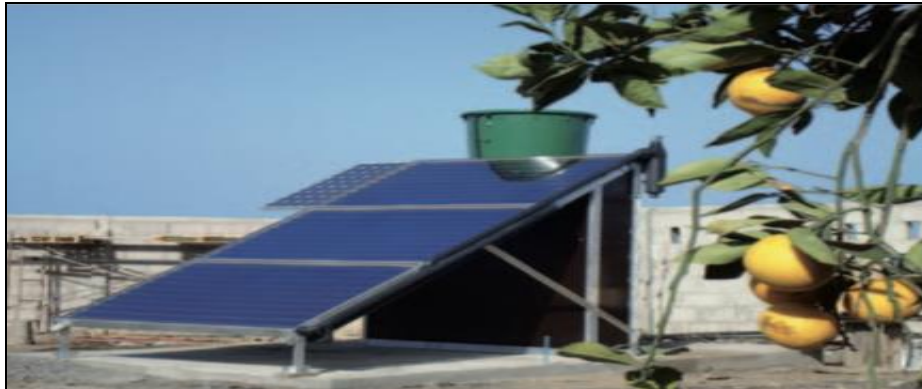
Figure 4: Membrane Distillation installed by SOLARSPRING GMBH
