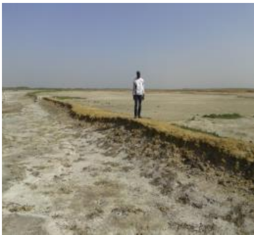
Picture 13 : Djimsane dike, clay backfill in left bank without crown, eroded
