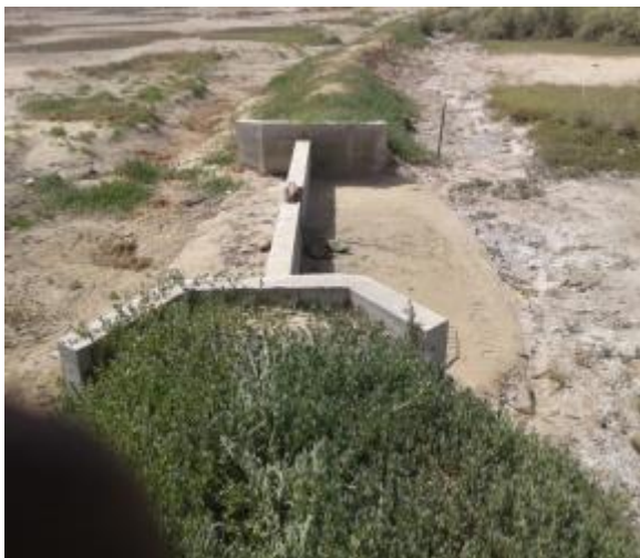
Picture 15 : Djimsane dike, which rudimentary spillway, equipped with a rusty metal valve, without rockfill makes it prone to washouts
