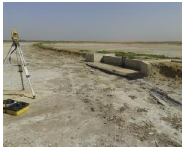
Picture 14 : Djimsane dike, clay backfill in right bank, without crown, and washouts at the base of the spillway
