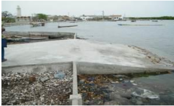
Photo 14: Dike made of RC plates
