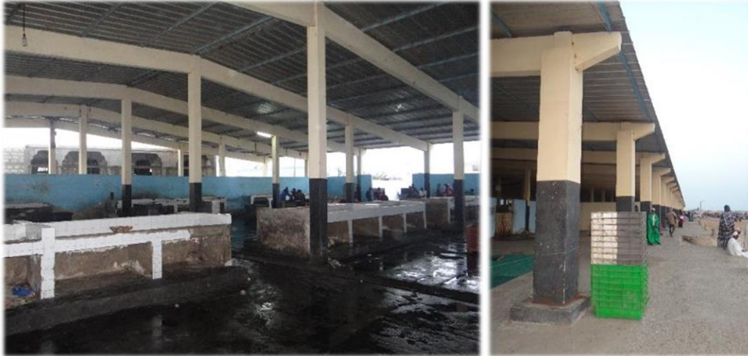
Photos 9 and 10. The pillars of the fishing dock were rehabilitated and the walls were painted.
