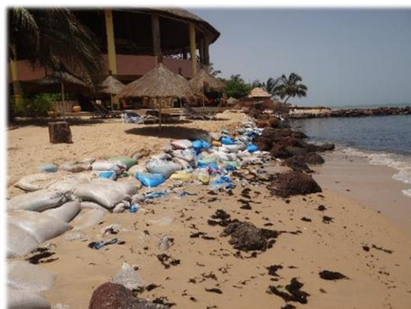
Photo 1. Several protection methods against coastal erosion implemented in front of a hotel in Saly.
