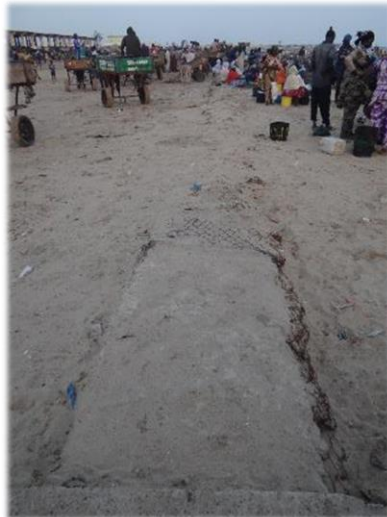
Photo 13. The dike and fishing dock almost entirely covered in sand. .
