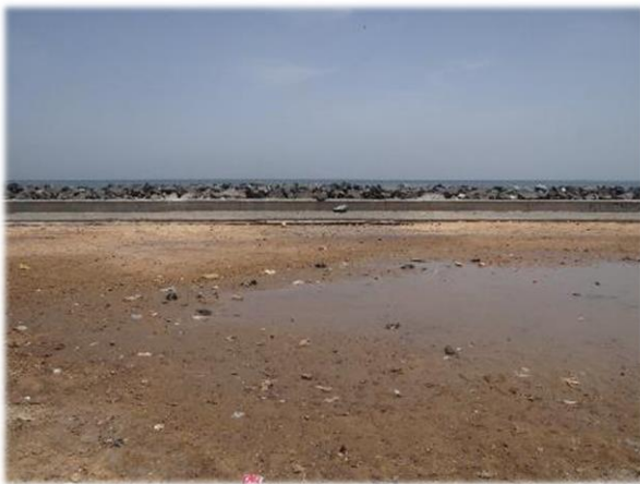
Photo 7. Stagnant water on the esplanade.
